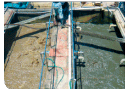
Operation in a aeration tank running condition
